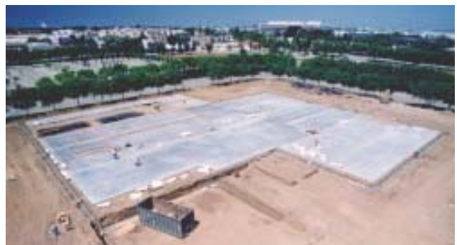
Floors and foundations are poured; the site progresses to the next stage.
